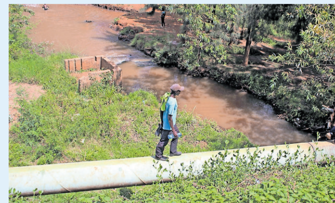
A man walks on a sewage pipe across Ruaka River near Thika Road at Allsoaps on March 13. KANYIRI WAHITO | NATION
